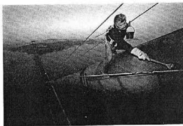
Figure 3 Some bridges are so big that painters take years to finish the whole structure. Then they have to start over again!
